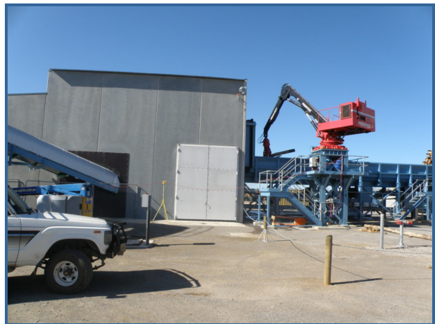
Doors in place at our client's premises after being fitted to the mill
